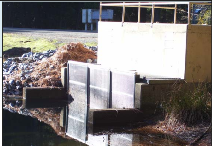
New intake screens at Walton Lake WTP
