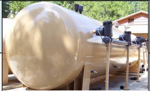
New filter at Walton Lake WTP
