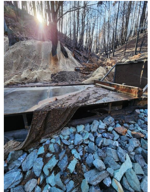
Storm water flowing over new flume cover purchased with grant funds.
