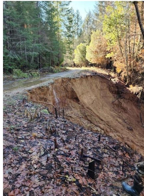
Road closure due to erosion being monitored by District crew.
