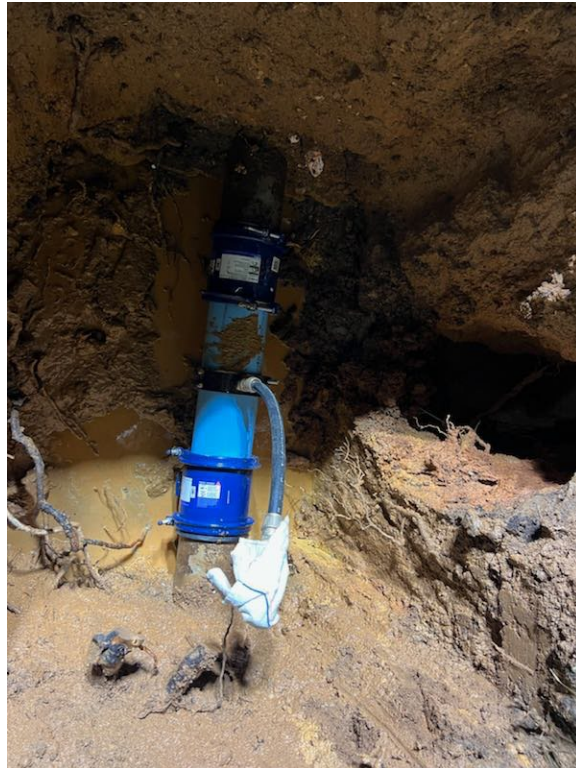
Mainline Break – 69 Labor Hours | Vac Trailer, Utility/Dump Truck, Excavator, Light Trailer
